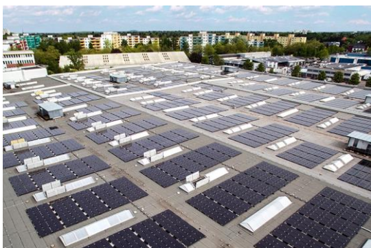
Photo: Solar rooftop at hybrid power plant Berlin-Marienfelde is the first pv system worldwide which operates at 1,500 Volt
