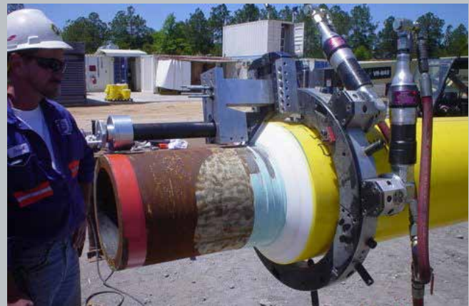
Our fast and versatile RBL split frame lathe was the ideal platform when a customer needed a light and reliable Coating Removal System that featured our custom designed form tooling bits.
