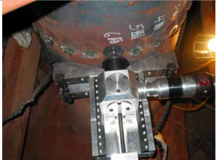
This heavy-duty machine above was designed and built to provide consistent depth and diameter cuts to remove socket welds in a very high-pressure heat exchanger header in a fossil power plant.
