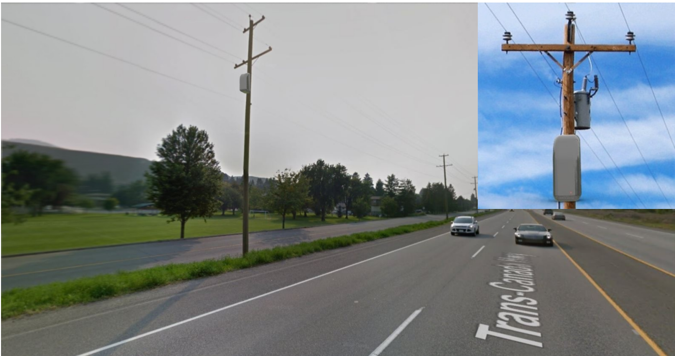
Image of utility pole with Reduction Tech mounted on it.
