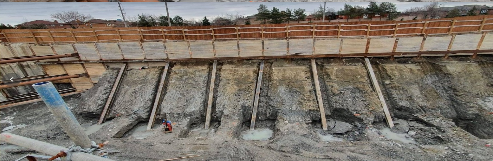
Excavation, Shoring and Caisson Piling Project for a Real Estate Project in Vaughan - Ontario
